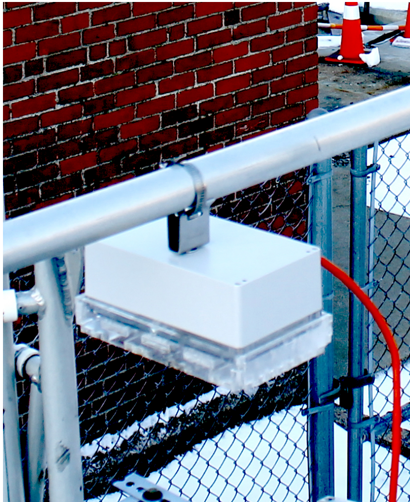
Figure 7: LearnAir Sensor installed at the MassDEP site, close-up
