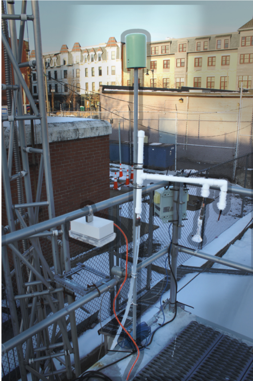
Figure 8: LearnAir Sensor (box on left) installation next to MassDEP inlet (top of pole on right)
